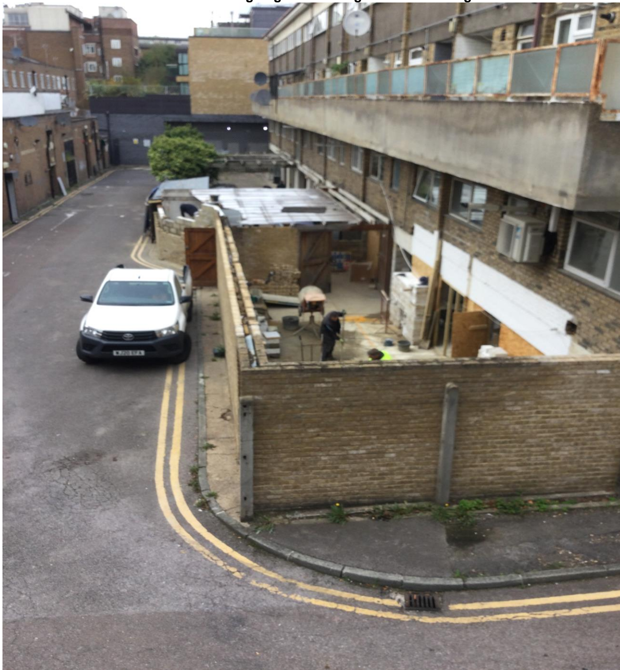
Rear elevation of Cervantes Court – garages at lower ground level being converted into 2 flats
